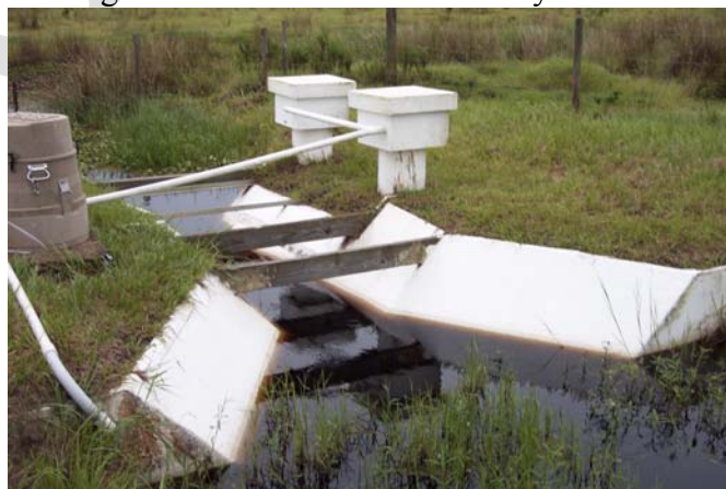
Figure 4. Photo of flume structure showing 1) two stilling wells (top center) containing shaft encoders to monitor water levels in the flume; and 2) an ISCO automatic water sampler (left) that collects samples just upstream of the flume.
