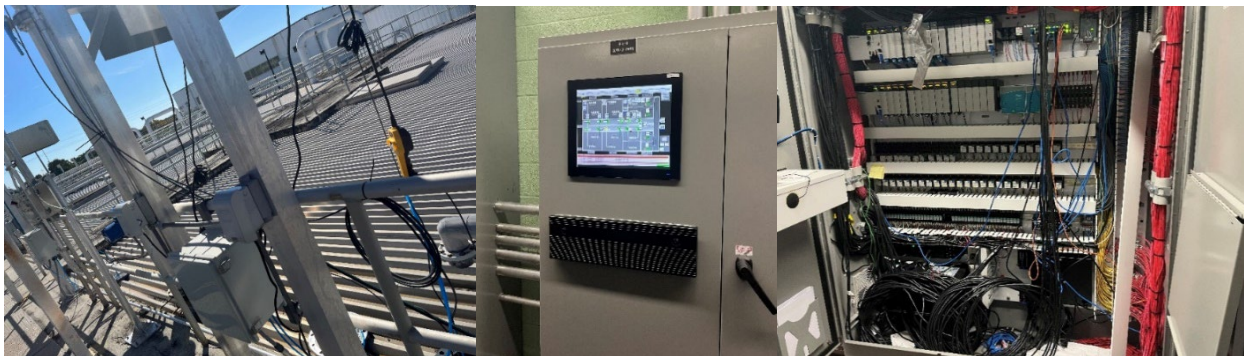
Above photos show the new aeration system for the South Central Regional Wastewater Treatment Plant and Disposal Board.
