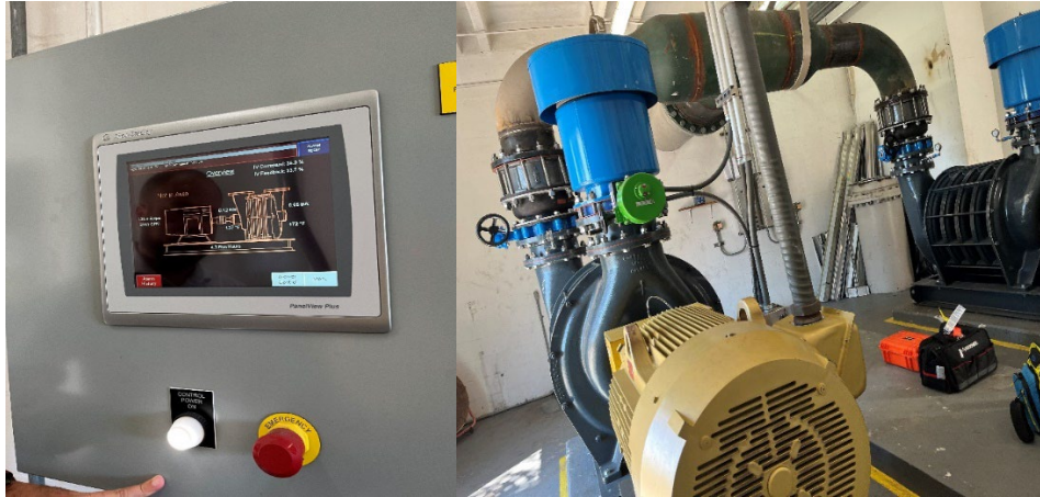
Above photos show the new blower system at Coral Springs Improvement District's Wastewater Treatment Plant.
