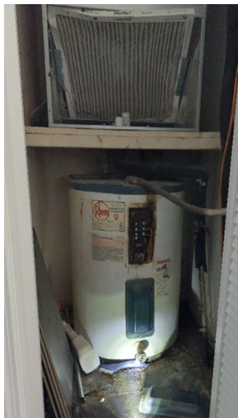
Old Water Heater
