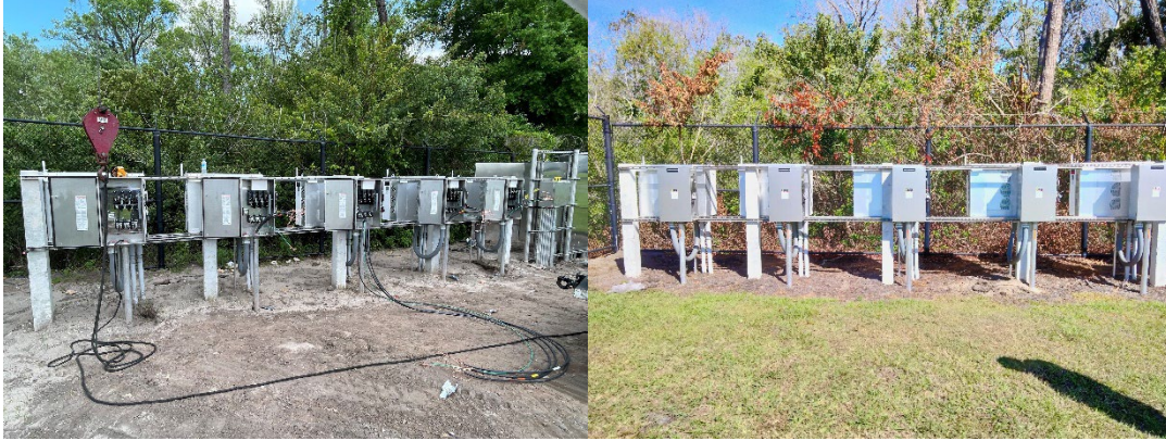
Above photos are pre- and post-install of AC disconnect switches on an existing inverter rack at the Regional Water Reclamation facility located in the City of Altamonte Springs, Florida.
